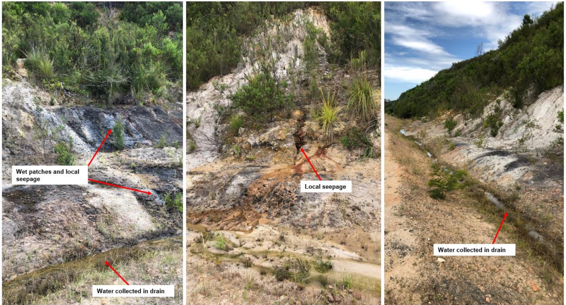
Figure 29 HHF Groundwater Seepage (February, 2021)
